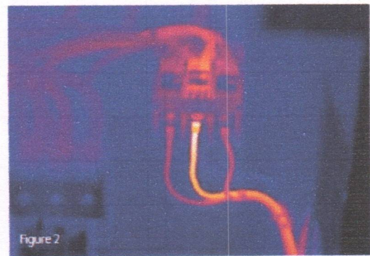
Figure 4 shows the same lead in operation at 320° F. The infrared image shows a possible loose connection or overloaded circuit.
