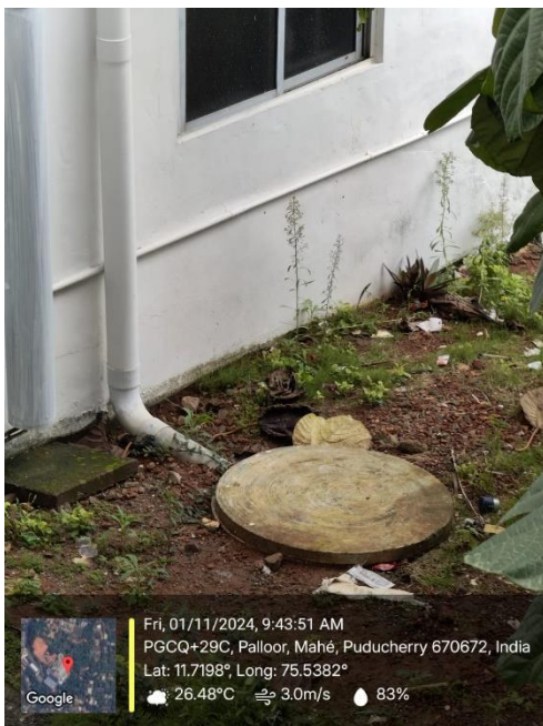
RAIN WATER HARVESTING
